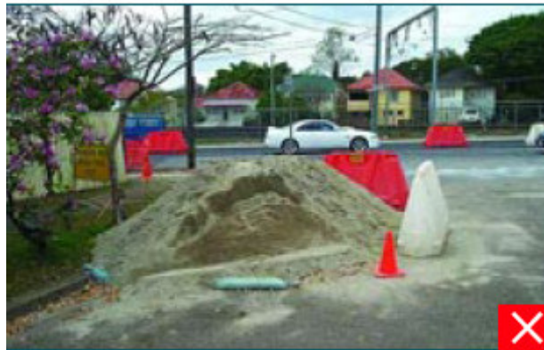
Stockpile not appropriately stored
